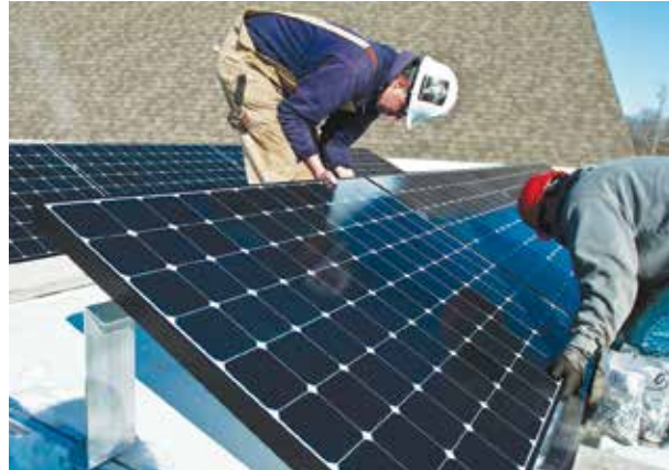
MGE has installed solar units throughout its service area, including this installation on the Aldo Leopold Nature Center.
