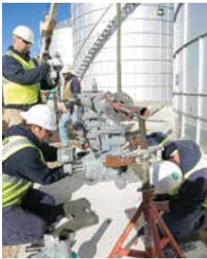
MGE crews install a natural gas meter next to a large grain dryer, which uses a significant amount of energy to dry crops for storage.
