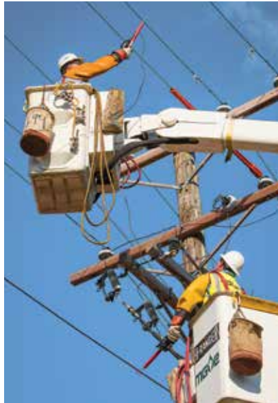
MGE electric line technicians make upgrades to our distribution grid as we work to keep our system strong.
