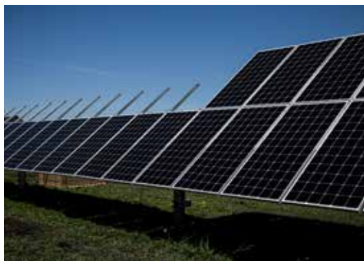
Construction of the 5-MW solar project at Morey Field in Middleton, Wis., is underway.
