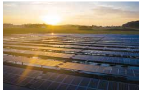
Morey Field Solar at Middleton Municipal Airport.
