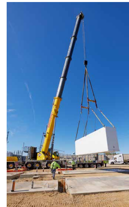
A future-forward electric grid is safe, reliable, adaptable and resilient. In the fall, MGE installed 7-MW batteries at three different locations across its distribution system. These batteries provide enhanced reliability and stability on our community grid from various points on the system.
