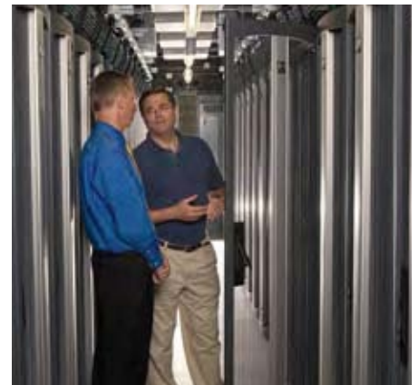
Don Larson (right), director of operations at TEAM Technologies, shows the data center to John Drury of MGE.
